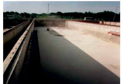
Effluent Treatment plant
